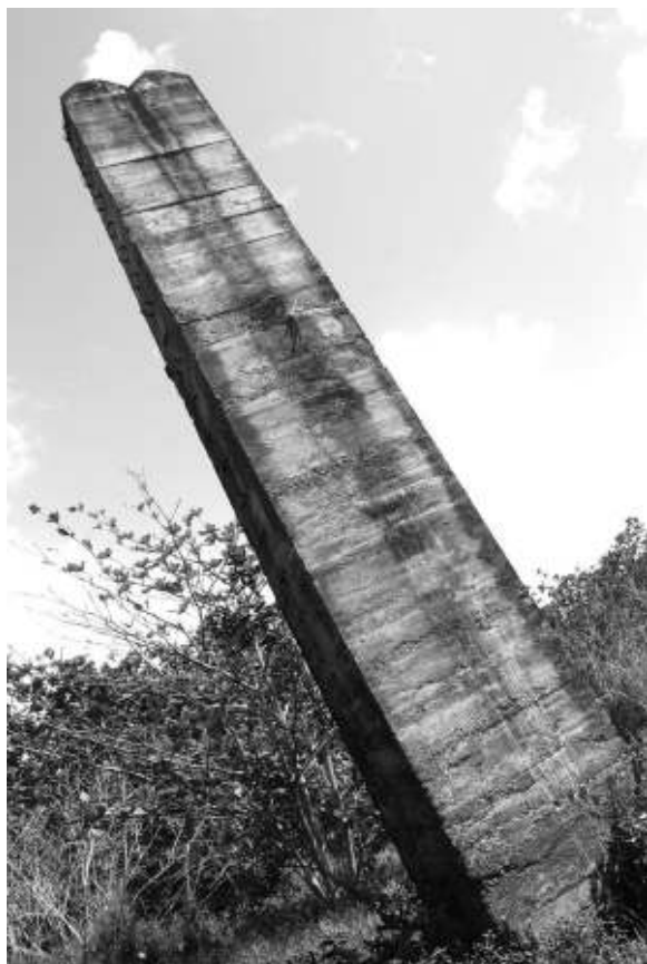
This concrete pylon was previously used to support a flume that spanned Oheo Gulch to transport sugar cane to the mill.
