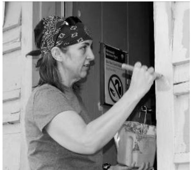
Volunteer Michelle Pellersels applies a coat of paint to Paliku cabin during a recent service trip.
