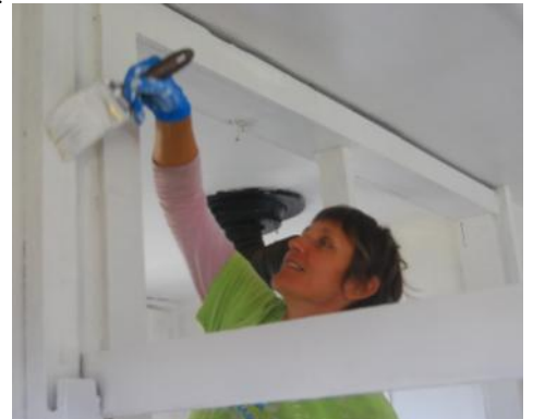
Above, Wal G. applies a second coat of paint on the interior of Kapalaoa cabin.
